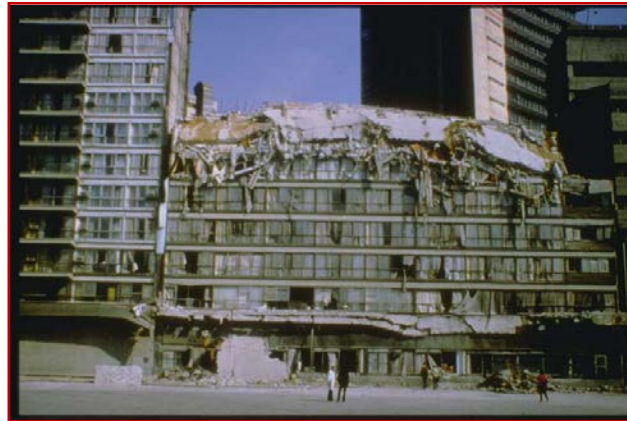
(FIG-12 : Collapse of adjacent building due to pounding effect in 1985 Mexico Earthquake)
