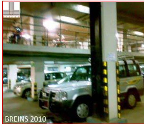
(FIG-10 : A newly built Commercial Complex with variation in Column heights within a Storey for double level Parking. Long, Slender Column is seen to be retrofitted with Steel Channels)
