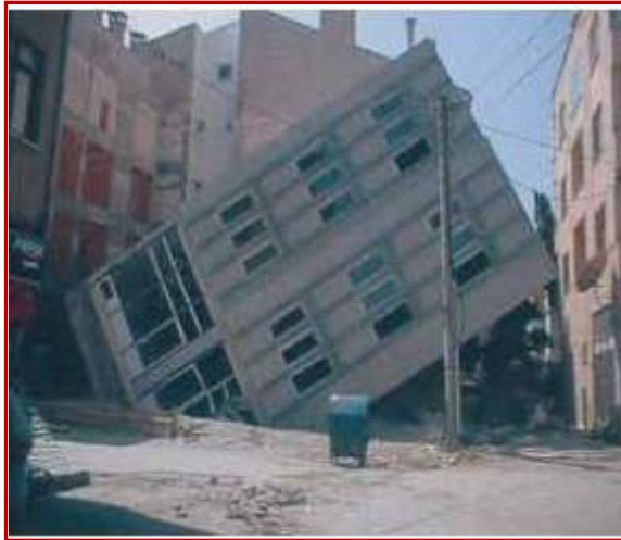
(FIG-13 : Four Storeyed RC Building overturned due to foundation failure in 2001 Bhuj Earthquake, India. Lifting of Raft Slab is seen in the Pic. )
