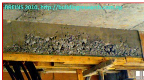
(FIG-19 : Inferior Concreting Works with Honey Combing and Holes; Design Capacity & desired Durability couldn't be achieved rendering weaker structures. Poor Quality Control)
