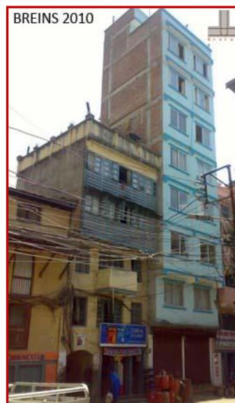
(FIG-11 : Newly built Nine Storeyed RC Building attached to Old Five Storeyed building. These Buildings may pound against each other due to difference in their vibrational characteristics; causing damage to the weaker one)
