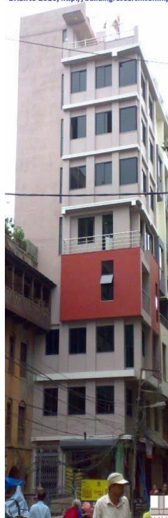
(FIG-14 : Slender Eight & Half Storeyed RC Building with overall height of around 90'-0" and front width of 15'-0" only; H/B ratio is 6 for this building )
