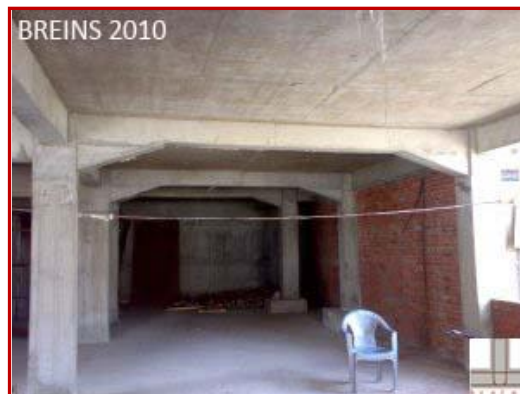
(Fig-5 : A Shear Wall-Framed Structured Building analyzed using modern techniques and designed to maintain Ductility)
