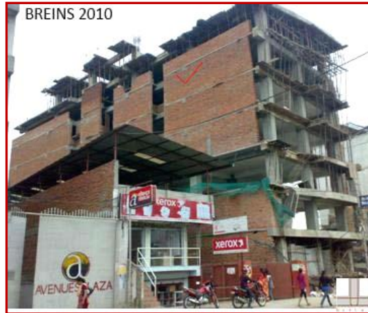
(FIG-17 : An Eight Storeyed Building including basement with 4” width brick walls along its boundary. The Brick Wall Panels were placed outside the Column Grids; directly on the Slabs, making it highly vulnerable in off-plane failure. Structurally designed & approved by the concerned Government Authority. But still lacks earthquake safety features as seen from the visual inspection)
