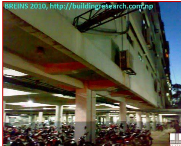
(FIG-9 : A Commercial Complex with Open Basement floor for the parking purpose. Almost all the Commercial Complexes have this feature in common)
