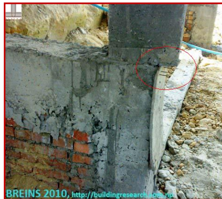
(FIG-18 : Column above Plinth Level misplaced by the offset of almost 3” outside; Column may fail prematurely at such places. Weak Technical Supervision; Similar problem as shown in FIG-16 above )
